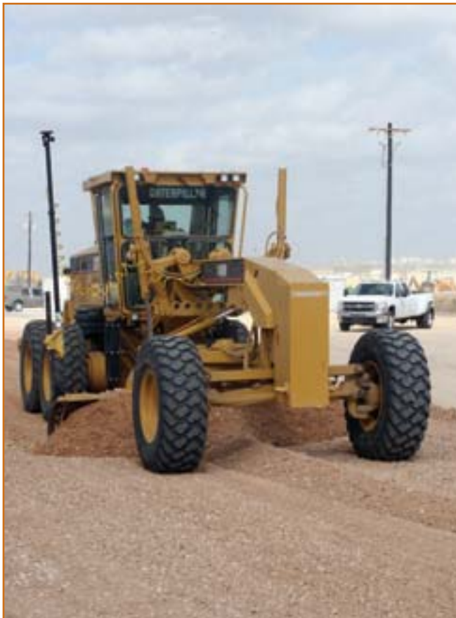
Tri-County's Caterpillar 140H motor grader is equipped with a Topcon GPS system and can grade base rock to within 0.10 foot.
